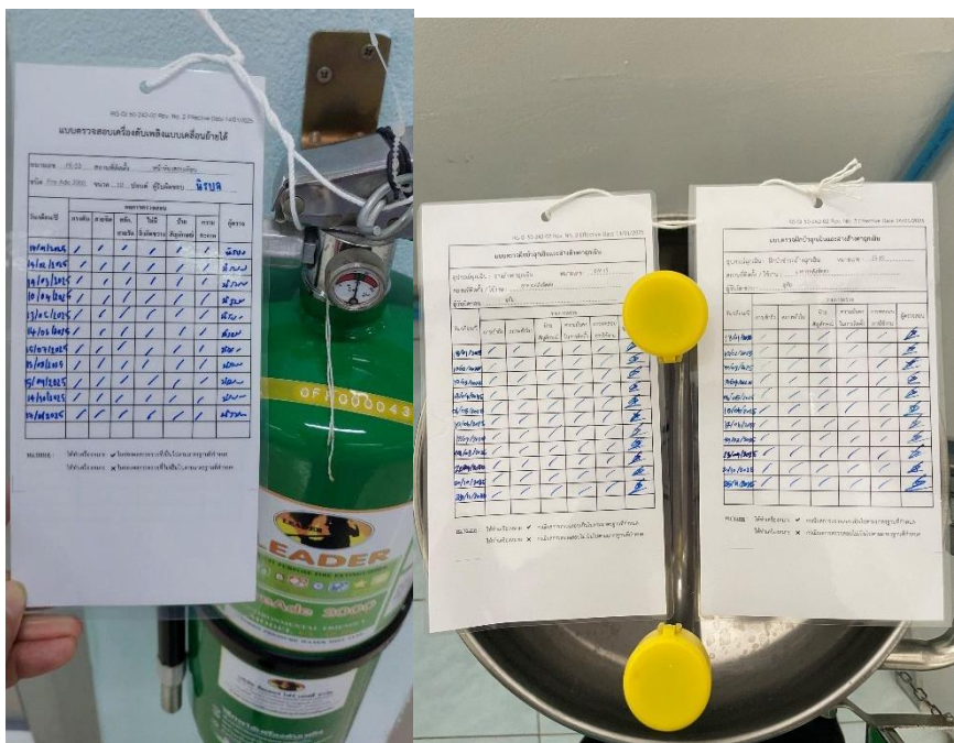
Image of emergency response equipment inspection
